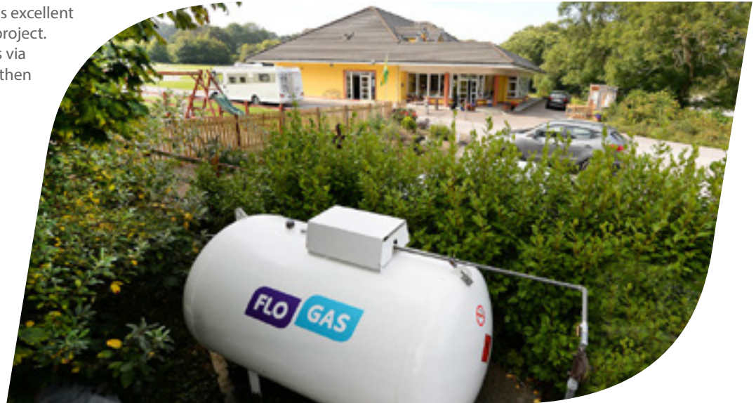
Flogas LPG tank
